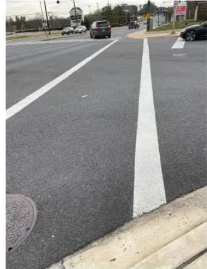
Security Lane (west) Lacks continental striping
